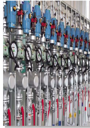
流量計 Flow meters
