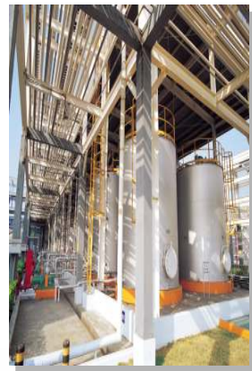
成品儲槽 Finished goods storage tanks
