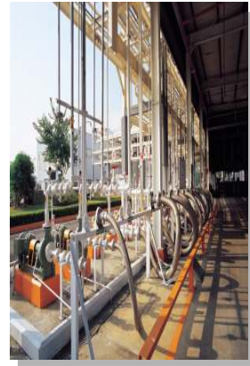
槽車入料 Tanker input materials
