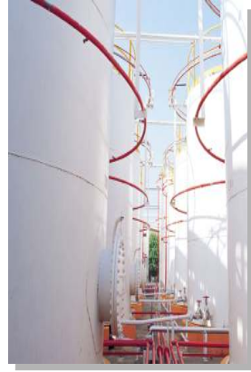
原料儲槽 Material storage tanks
